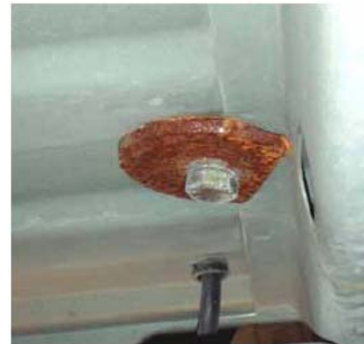
Figure20. Load-spreading washer located under vehicle bed
